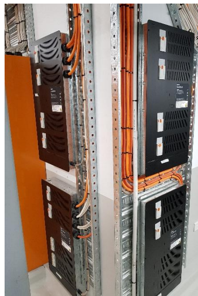
Wall mounted controllers
