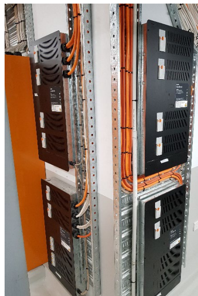
Wall mounted controllers
